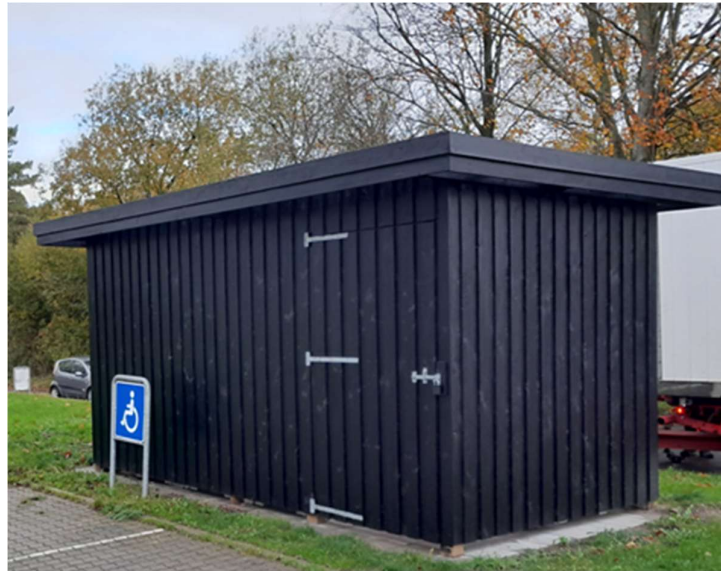
Figure 12. Shed with Huawei battery and inverter.
