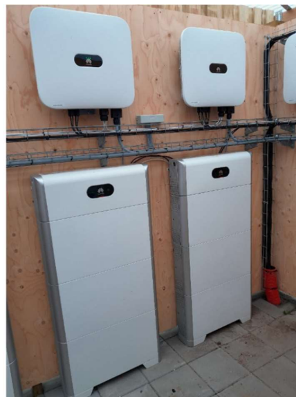
Figure 13. Huawei battery and inverter.
