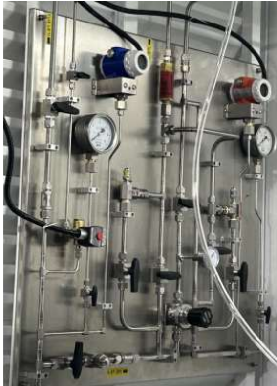
Figure 15. Hydrogen busbar system
