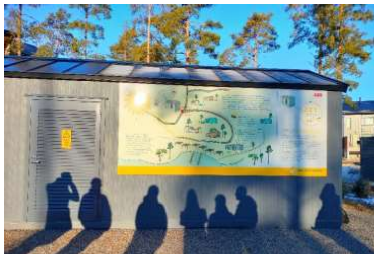
Figure 47. Smart distribution substation. PS#7
