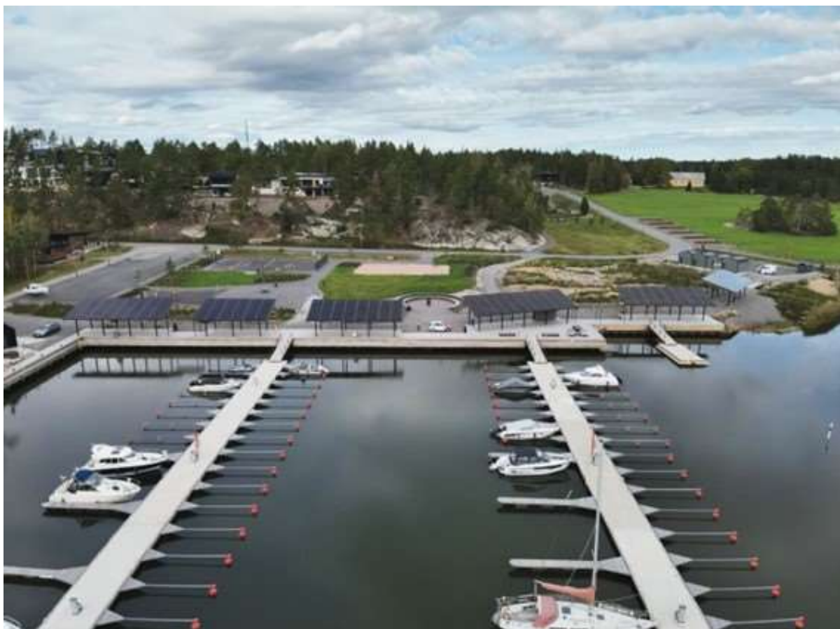
Figure 45. Bi-facial PV Modules based installation at Naantali pilot site. PS#7
