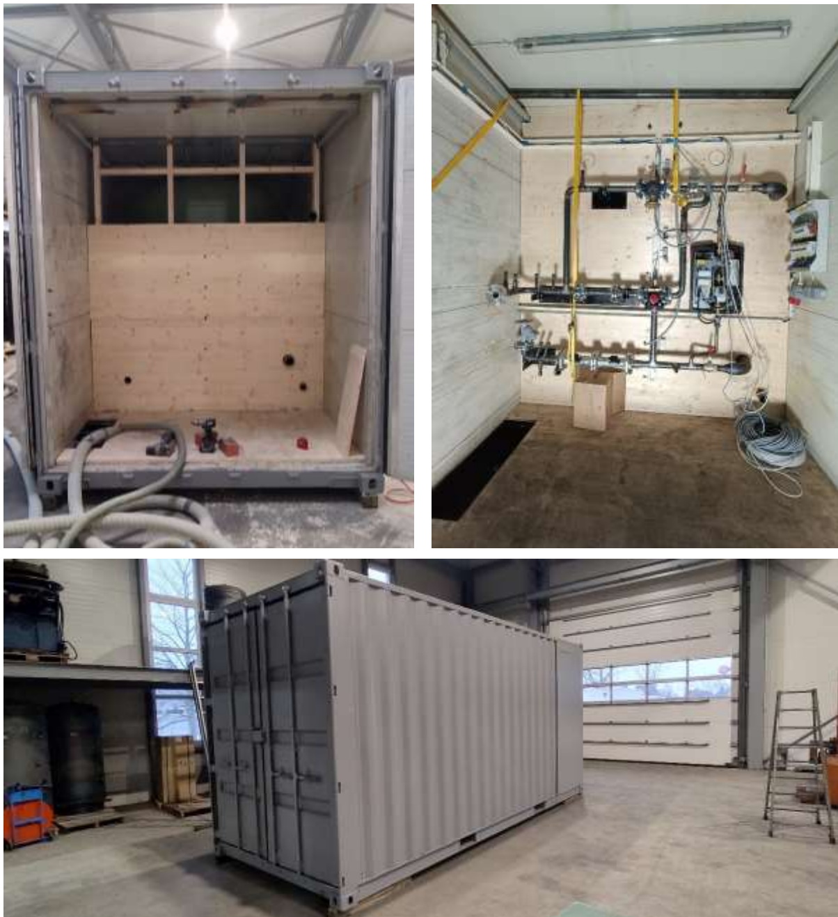
Figure 52. Cladding and piping and container of the DH-buffer tank
