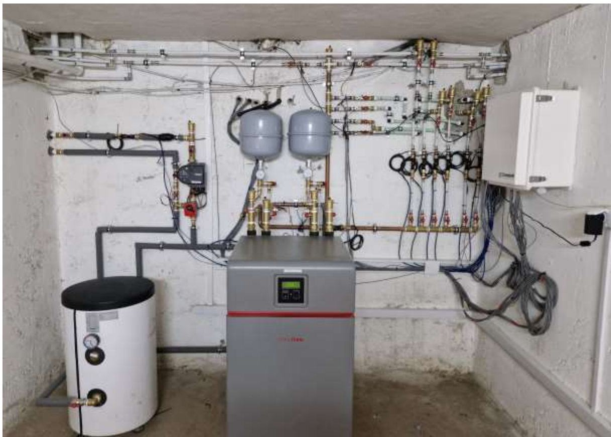
Figure 22. Heat pump technical room
