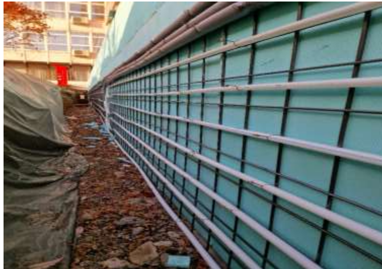
Figure 18. Exterior GeoWall system with Pe-Xa pipes
